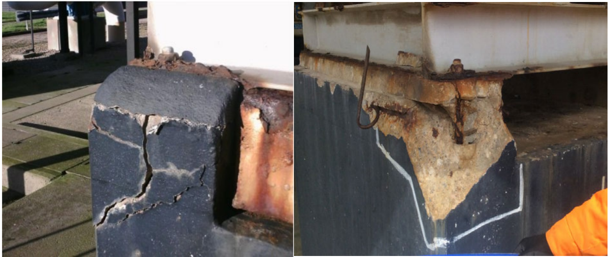
Figure 7: Plant 2 Aftercooler fan concrete support plinths: cracking, corrosion and loss of section
