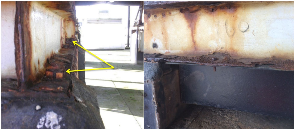
Figure 8: Corroded anchor bolts and steel mounts
