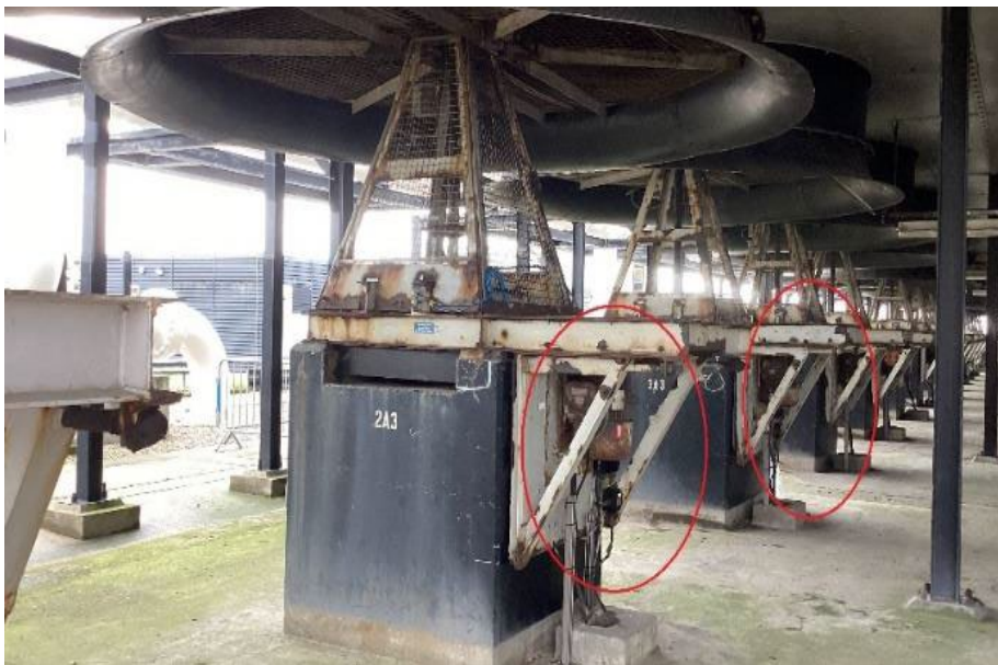
Figure 10: Plant 2 Aftercooler motors
