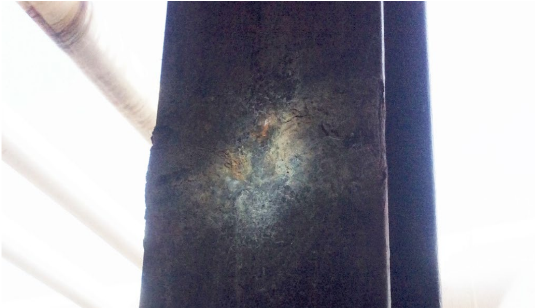
Figure 9: Steelwork column bulging (at 2/3rds height) due to severe corrosion.
