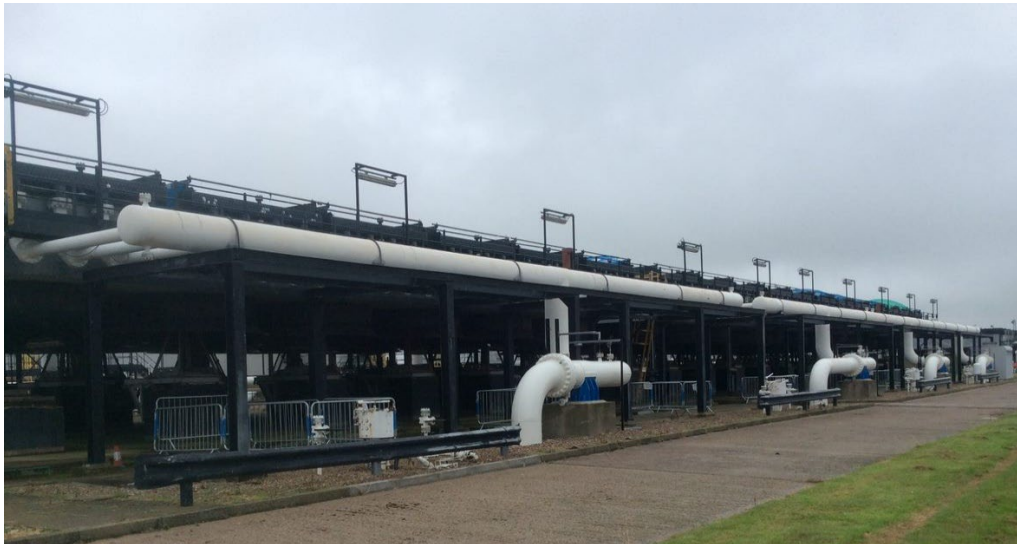
Figure 6: Plant 2 Aftercooler Outlet
