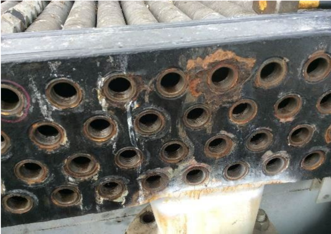
Figure 11: Header plug sheet corrosion
